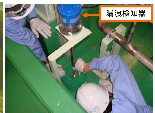
PCB漏洩検知器の点検
